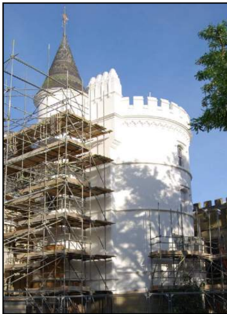
The Beauclerc Tower, now repainted in brilliant white. Photograph by Richard Spires
