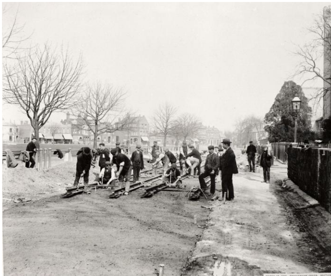
Laying tram tracks on Hampton Road on 18 th March 1902. The tower of Holy Trinity church can just be made out on the right
