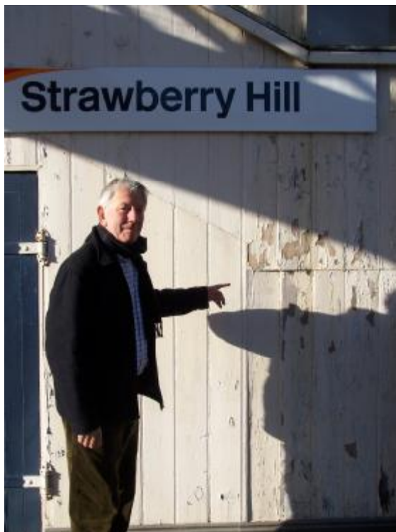
Joe Brett points out the poor state of paintwork. Much of the wood cladding around the foot bridge is rotten.
